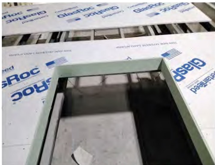
TBM-3 Thermal Break in window RO to reduce “flanking” around window frame
